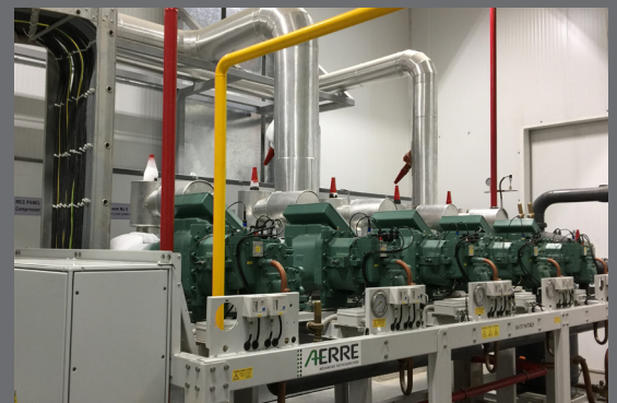
Refrigeration Rack System
